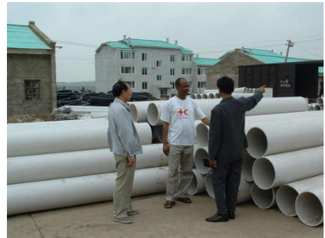
DPRK Red Cross trained local technicians to install water and waste water pipes and fittings.
